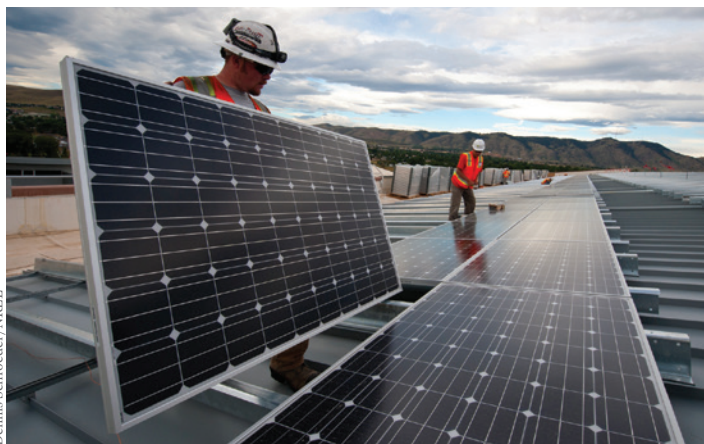
Federal infrastructure policy should prioritize modernizing the transmission system and enabling technologies such as offshore wind and battery storage, which will unleash vast amounts of renewable energy while driving economic development and creating high-quality jobs.
