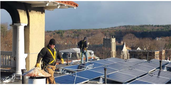
In 2015 the Laconia Housing Authority gave their 100 year old Strafford House facility a deep energy retrofit with the help of funding from the Community Development Financing Authority. The project included comprehensive air sealing and insulation, triple pane windows, LED lighting with smart controls, low-flush toilets and a 35kW rooftop solar array. (NHCDFA)
